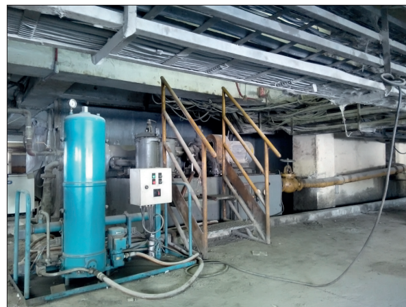
Finish Grinding Mill No. 1, Gearbox at Lafarge Republic Inc., Iligan Cement Corp. with CJC™ Fine Filter HDU 27/108 installed
